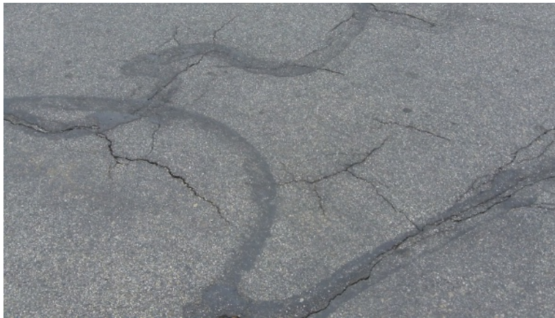
Figure 4. Photograph from the street cracks problem-finding item.
