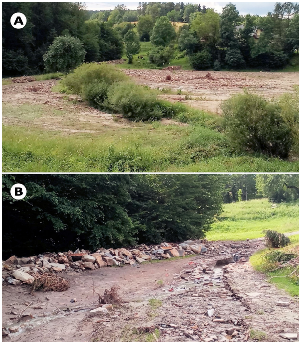
Fig. 8. A – Overview of debris-flow cone No. 2. The central (mid fan) sector of the cone shows an accumulation of coarse debris lobe, whereas the marginal zones are composed of gravelly sandy sediments. B – The apex part of debris cone No. 2 with incised channel. Sandstone blocks and boulders, up to 90 cm in diameter, accumulated at the mouth of the forested V-shaped valley.
