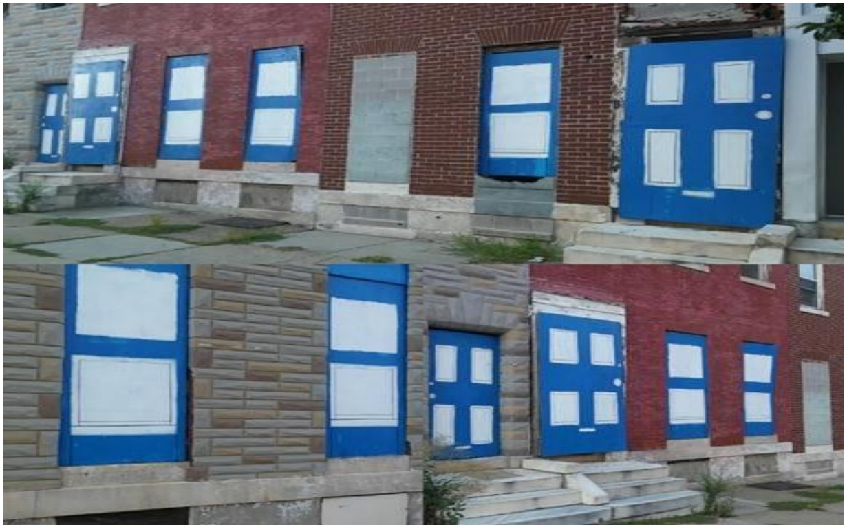
The plywood boards on the vacant houses on the 1500 block of West Lexington Street. Photographs by Kenneth Clemons, August 20, 2016.
