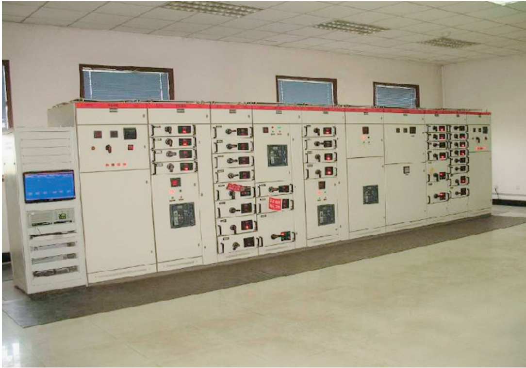
Fig 5.5 the power supply and distribution system of BPL long wave time service station
