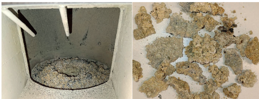
Fig. 3. Slag formation inside of burner (left) and taken out of boiler (right) from reference tests.
