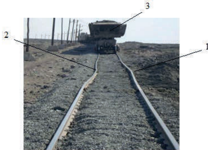
Fig. 1. Railroad track on a waste heap. 1 – buckle of rail track; 2 – subsidence of ballast layer; 3 – wagon.
