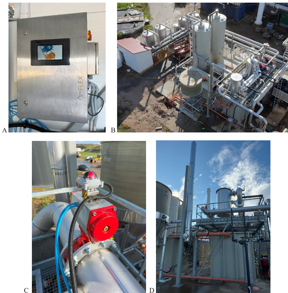
Fig. 8. Auxiliary equipment items: A gas analyzer (see Fig. 8A), pipeline installations (see Fig. 8B), valve kit (see Fig. 8C), as well as biofilter (see Fig. 8D).
