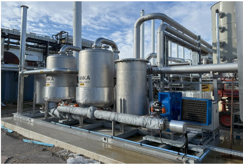
Fig. 6. Siloxane removal unit.
