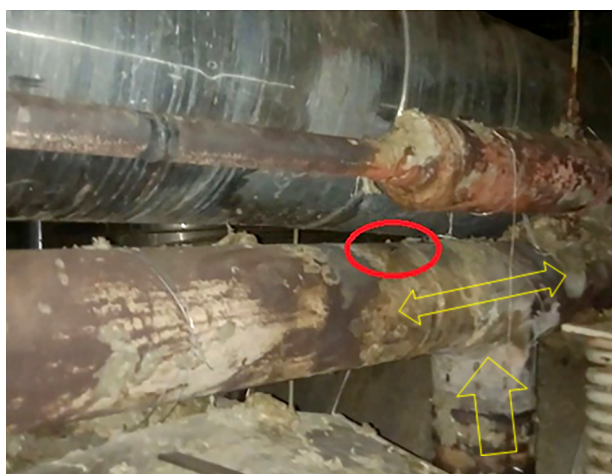
Fig. 1. Leaking on steam-pipe – red ellipse
