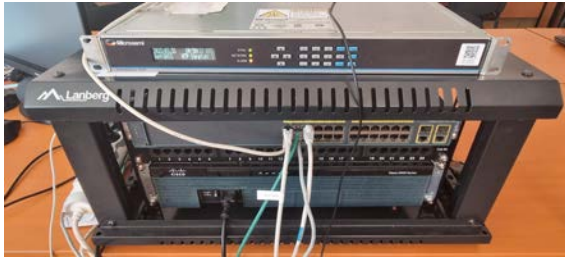
Figure 2: Syncserver S600 (up), Cisco Switch (middle) and Cisco Router (down)
