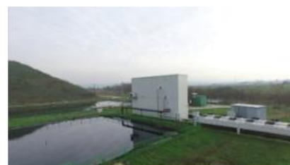
Biogas capture station
