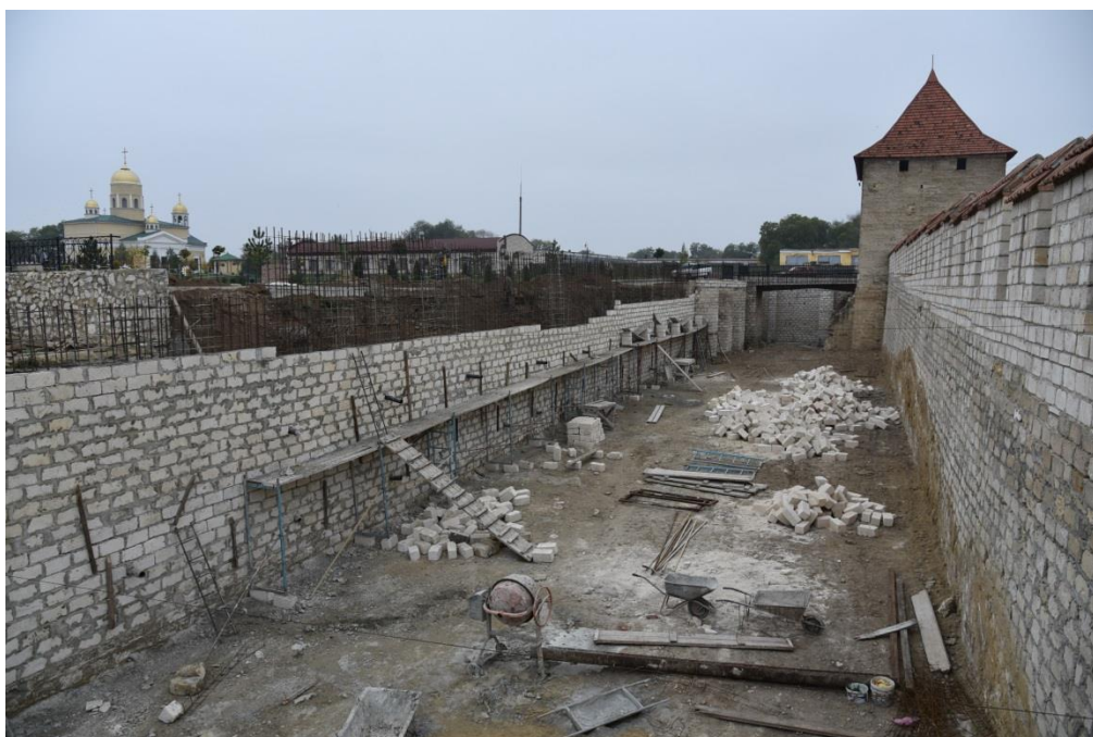
Figure 10. Construction of some parts of the walls around the Tighina-Bender fortress (author's own photo, 2019)
