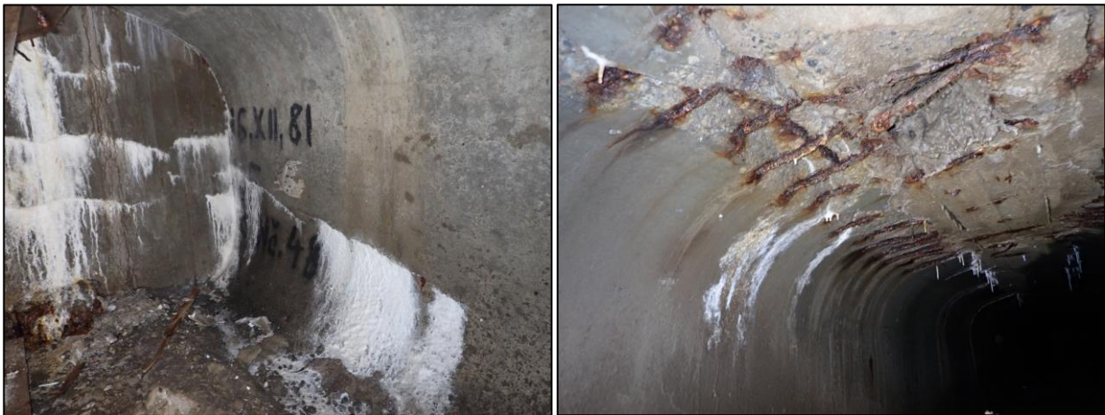
Figure 4: Significant active water leakage into the cells between the I-73 girders. Visible surface degradation of the concrete and exposed reinforcement. Observable paths of prestressing reinforcement (cracks and leachates)
