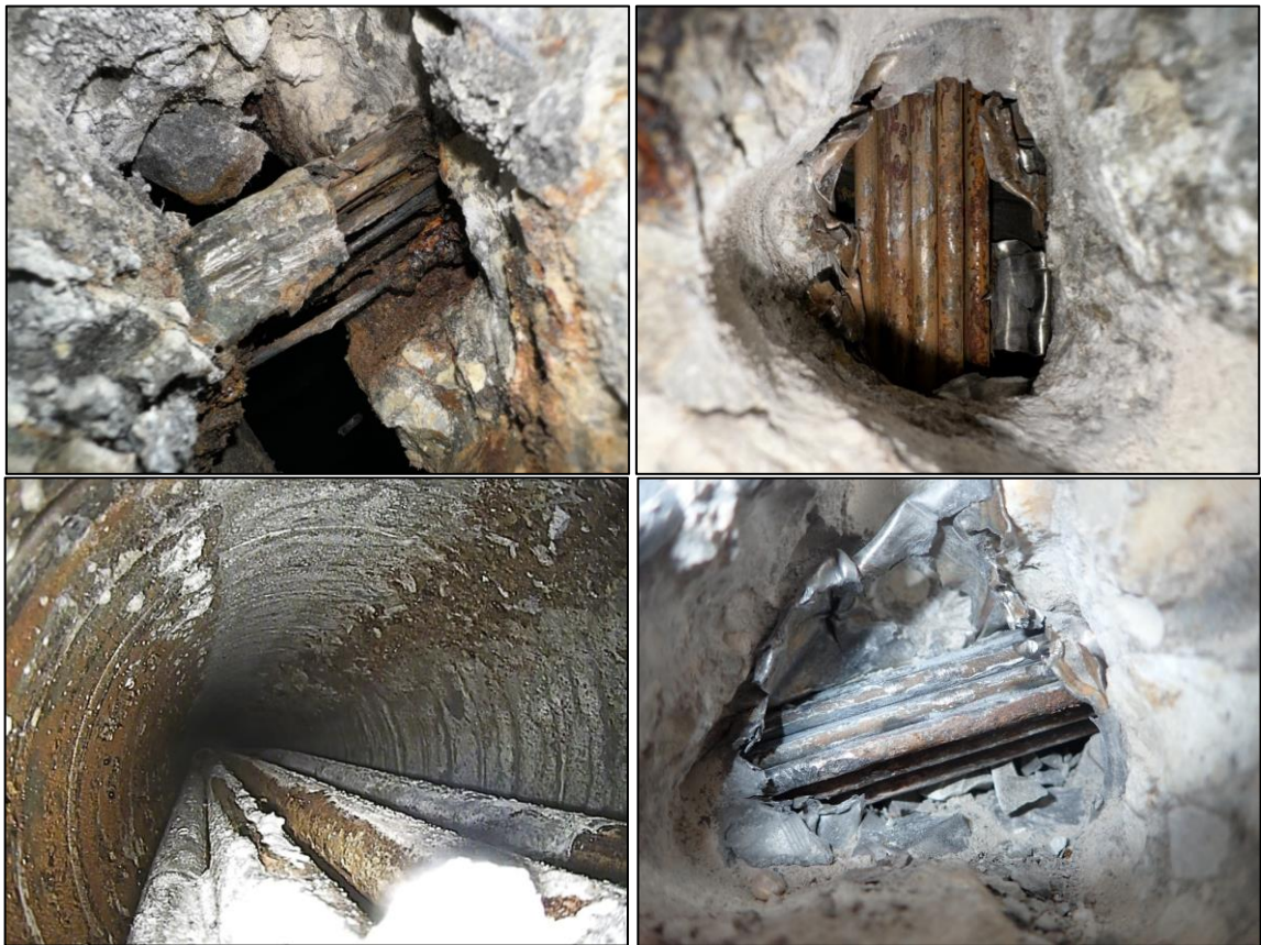
Figure 5: Presence of non-grouted tendon ducts and corrosion of prestressing strands and wires
