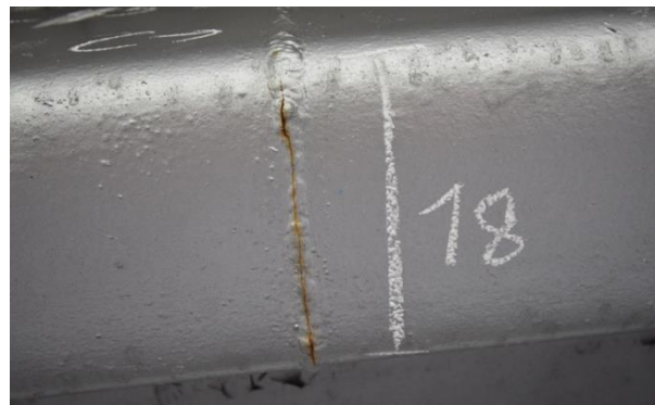
Figure 4: Crack in the weld at the longitudinal stiffener splice
