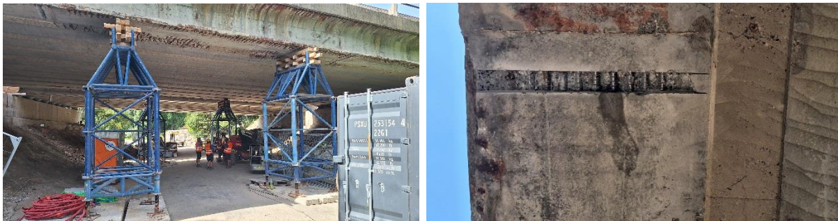
Figure 10: Damage to the edge girders before next measurement
