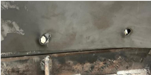
(c) Bearing damage of sheathing-Experimental results
