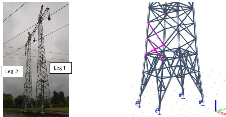
Figure 10: Tower No. 906 on line V423 – Brno-Chrlice, damage on the right
