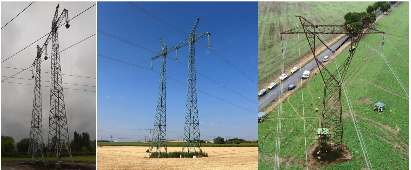
Figure 2: Measured structures from left to right: portal no. 906 (V423), portal no. 912 (V423), cat-type no. 28 (V470)
