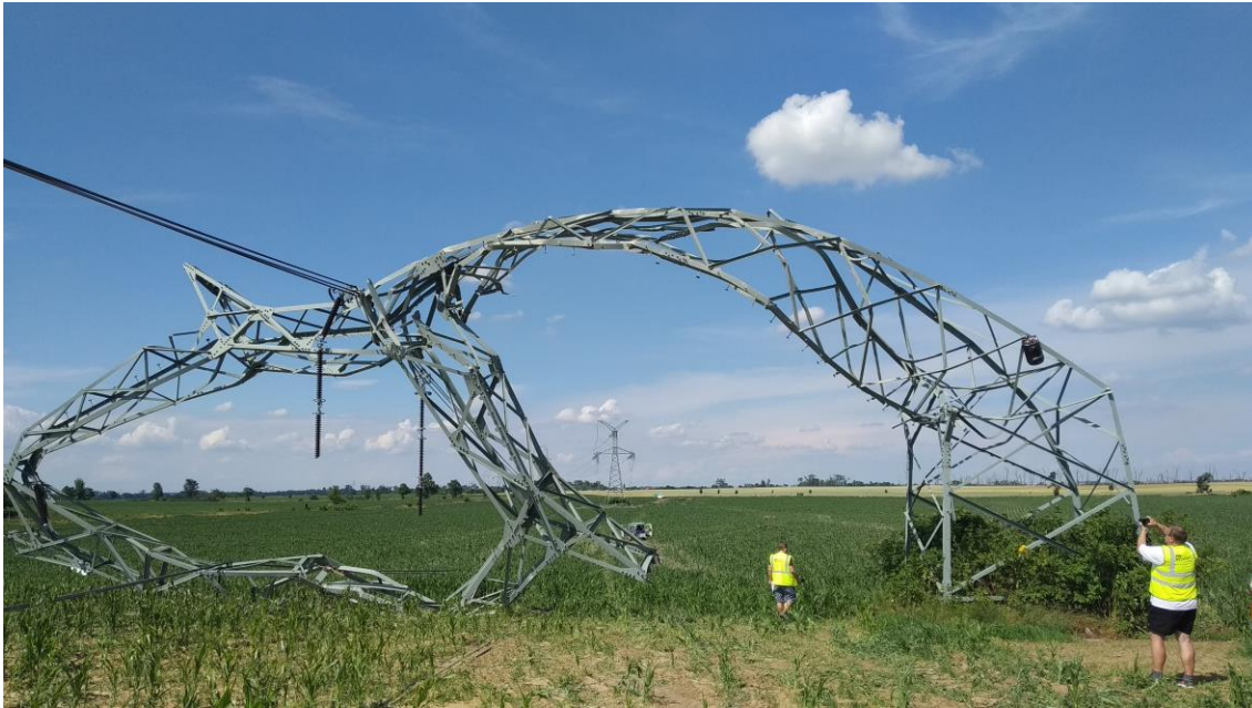
Figure 1: Collapsed Delta tower after the tornado in South Moravia
