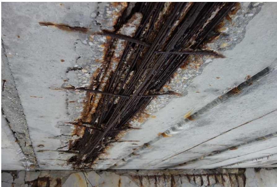
Figure 7: View of corroded prestressing wires
