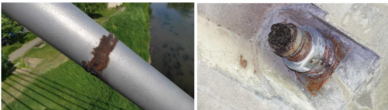
Figure 8: Results of visual inspection: a) corrosion of external sheath joints, b) corrosion damage to the protective coating system of the anchorage and missing anchorage cover
