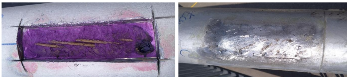
Figure 12: Cut-through probe through the stay cable sheath on the bridge in Židlochovice: a) indicative pH test, b) sealing with a welded steel patch
