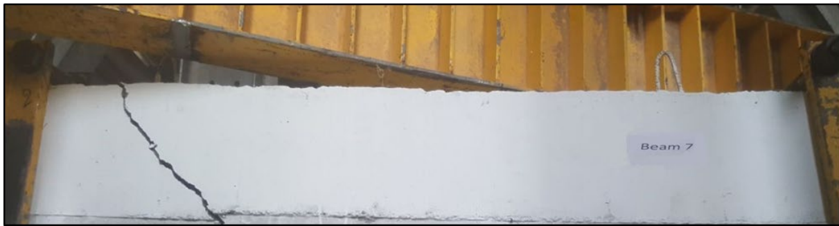
Fig. 18 Cracks Pattern in Beam BSGFT
