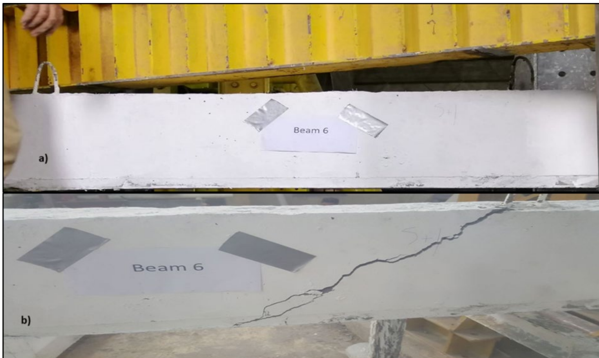
Fig. 17 Cracks Pattern in Beam BSHFTb a) before loading, b) after loading
