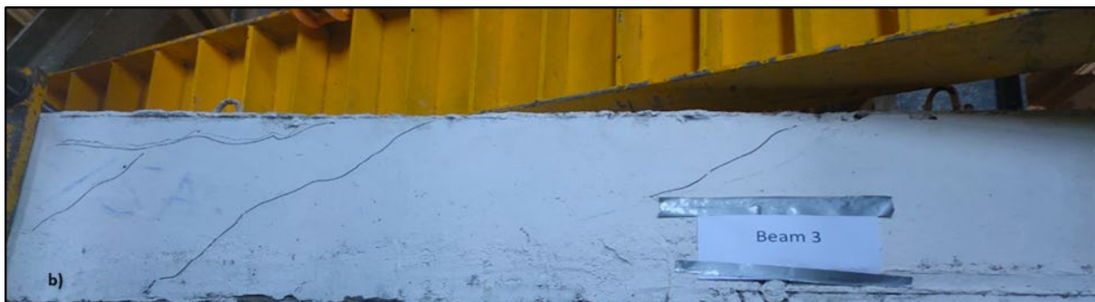
Fig. 14 Cracks Pattern in Beam BSSFF a) left side, b) right side
