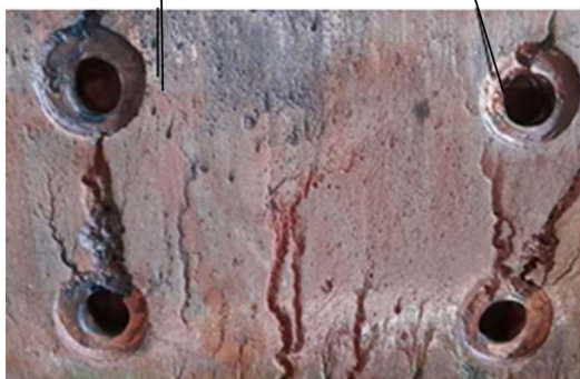
Figure 16. Galvanic corrosion in the area where the anodes are clamped with bolts
