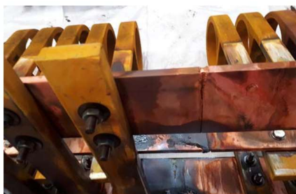
Figure 11. Copper bar breakage in crevice corrosion
