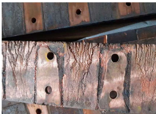
Figure 15. Galvanic corrosion of the copper bar
