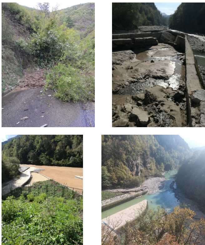
Figure 8: Destroyed access road to HPP Jablanica power house (up); The walls and protective layer of the outlet channel HPP (down).
