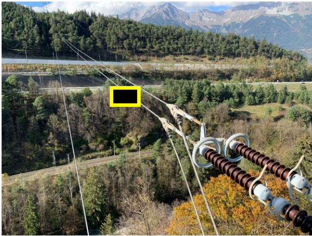
Figure 1: Location of a DLR Sensor on a 220-kV-OHL (marked by the yellow box)
