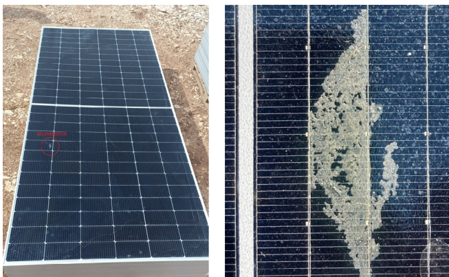
Figure 8: Example of delamination in the PVPP “Zvizdan”
