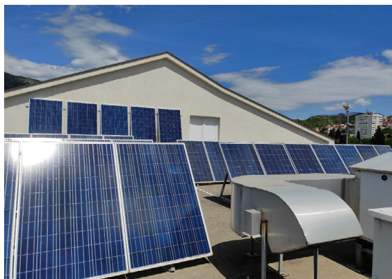
Figure 3: Solar panels on the south side of the roof
