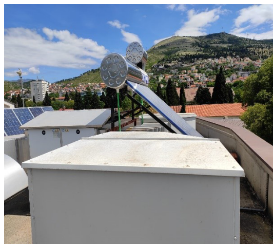
Figure 5: Solar collectors on the roof
