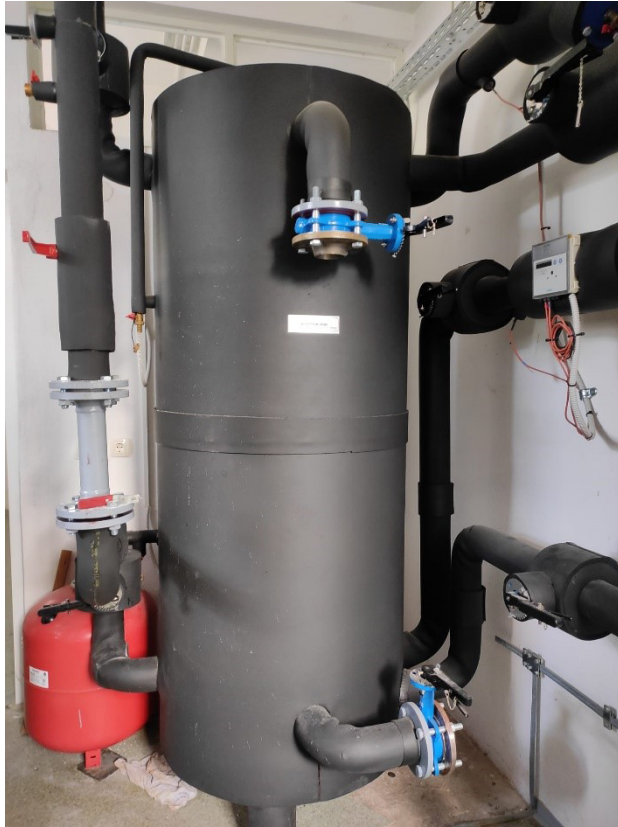
Figure 6: Systemair heat pump at the Faculty
