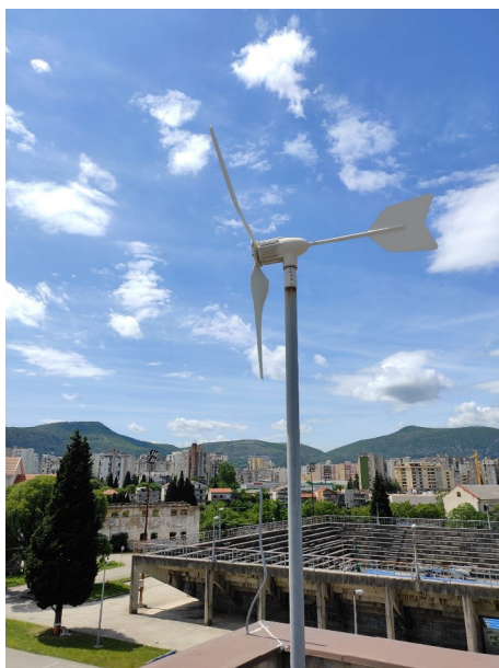
Figure 4: The wind turbine on the roof
