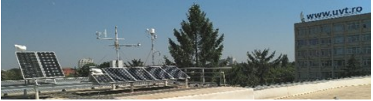
Figure 1. FORPV experimental setup located at the Solar Platform at West University of Timisoara
