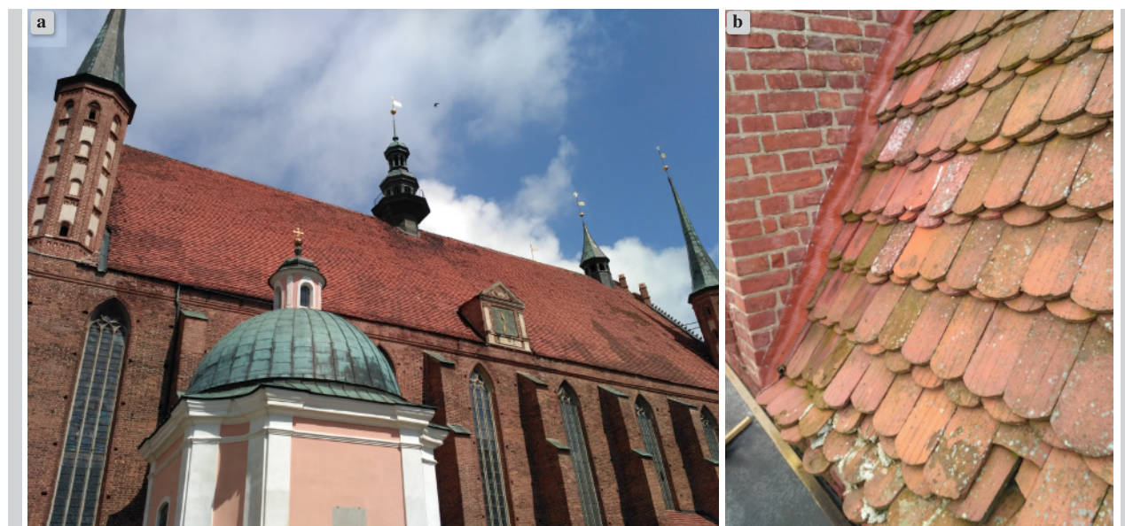
Figure 2. Condition of preservation of the south nave roof slope a) overall view b) zoomed area (visible broken and destroyed roof tiles)
